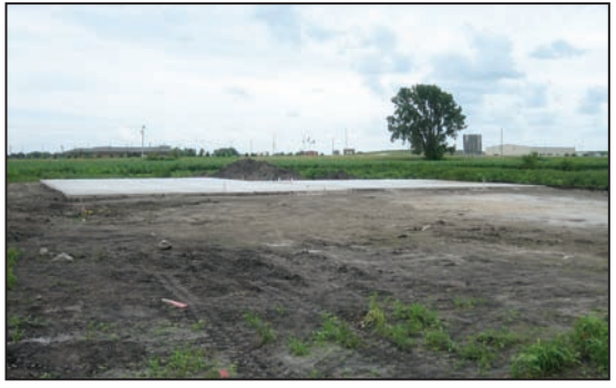
The cement footings and construction pad have been poured and await construction.
