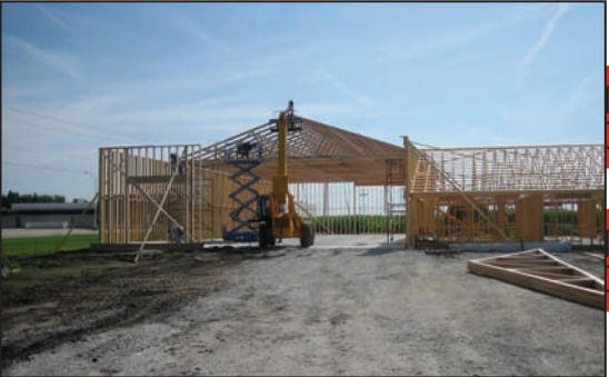
The warehouse walls are in place and the trusses are going up!
