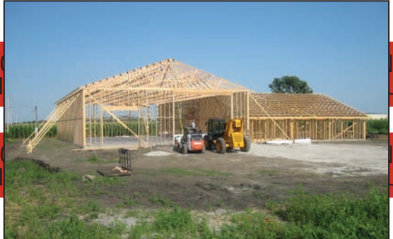
The office and warehouse are now framed and trussed. Once complete, the building will provide space for a pet-food distributorship and possibly another business in addition to the AASV.
