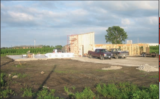
The office walls are up! The taller wall divides the office from what will be the warehouse.
